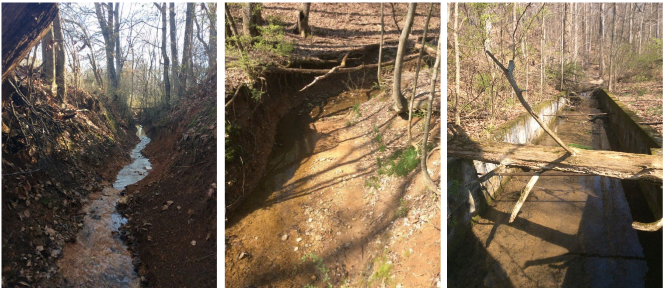
Figures 5-7. Examples of severe bank erosion and channel alteration in the headwaters of Turkey Creek.
